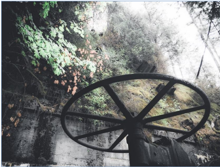
A large valve associated with the penstocks of Powerhouse No. 2. Chloe Tu photo.
